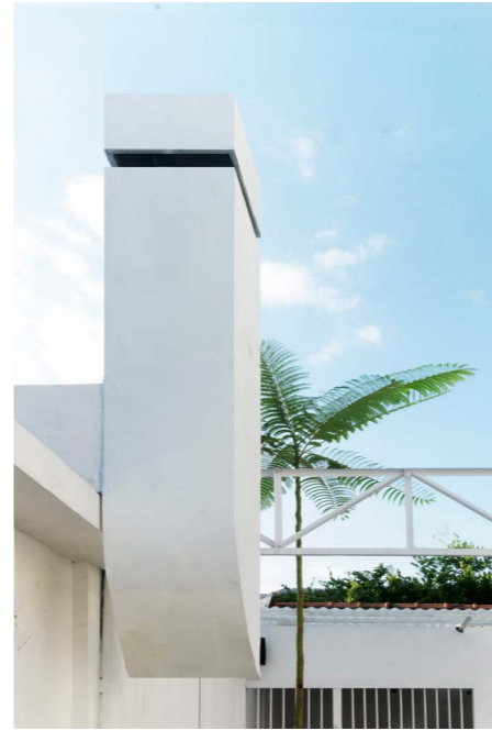
additional exhaust chimney was added in order to improving the exhaust system for each fnb tenant that using the existing building
