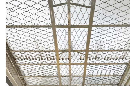
tranlucent roof at the carport
