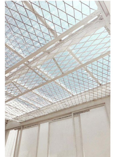
tranlucent roof at the carport
