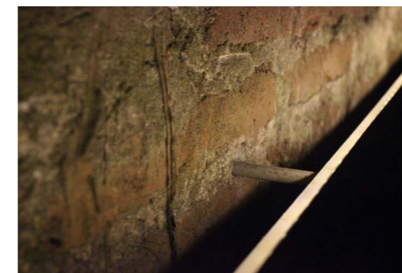
detached joint for lighting system
